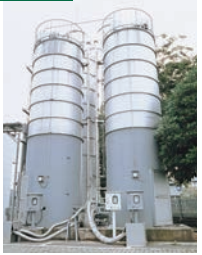
Material Storage SILO
