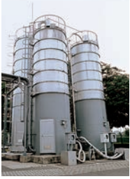
Material Storage SILO
