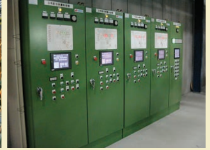
Powder and granule mixing system panel
